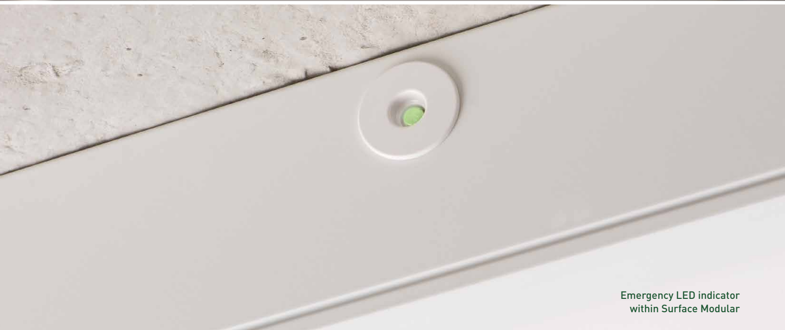
Emergency LED indicator in suspended ceiling tile
